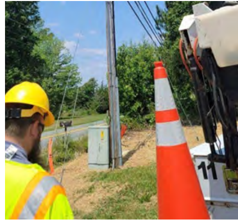
Underground fiber optic network construction in West Piedmont Planning District Commission SLFRF Funded Project.
