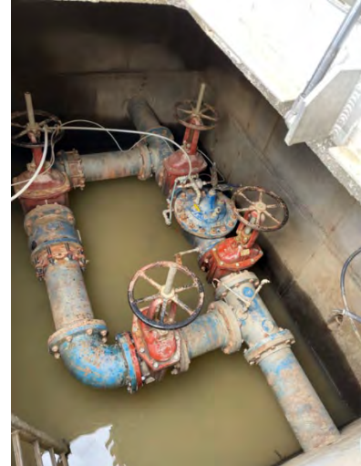
Flow control valve vault which allows water to flow into town from near the spring and the upper side water storage tank.
