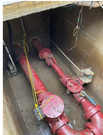
Altitude valve vault at one of the town water storage tanks. This tank would not fill completely.
