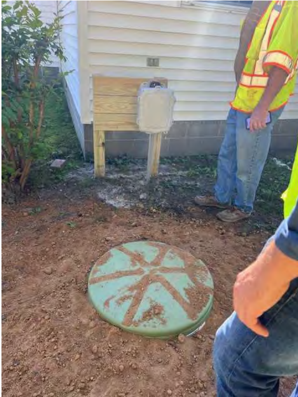
Town of Exmore (4400401): Residential E-one grinder pump station and control panel installation.
