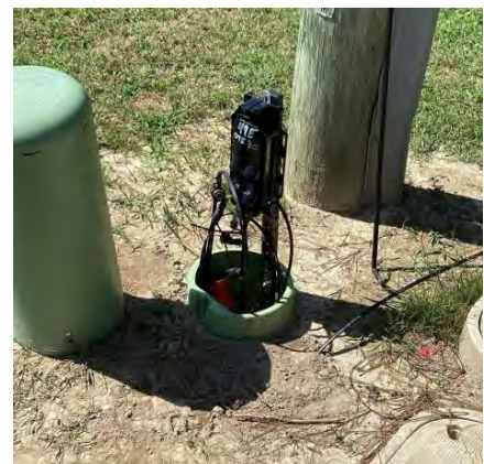
A broadband network terminal, where lines are connected between line extensions to households and mainline broadband infrastructure
