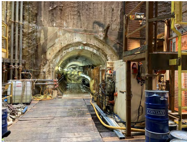
Alexandria Renew Enterprises (4400101): View inside the Waterfront tunnel shaft looking towards constructed portion of tunnel.
