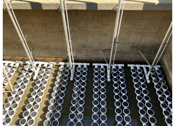
Wise County PSA (4400301): New aeration diffusers, activated sludge tank
