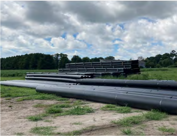
Hampton Roads Sanitation District (4400205): Force main storage for installation from Accomac to the Onancock STP on the Eastern Shore.
