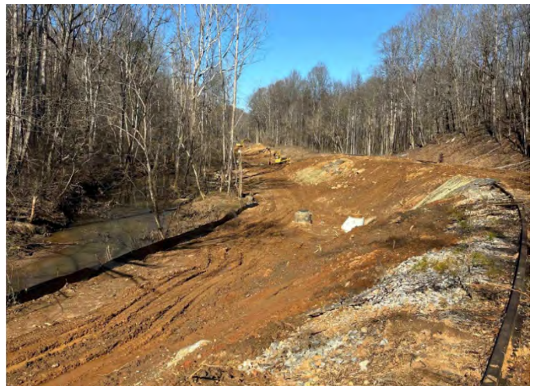
Martinsville (4400207): Jones Creek Interceptor work looking upstream from railroad tracks to the upstream extent of construction.
