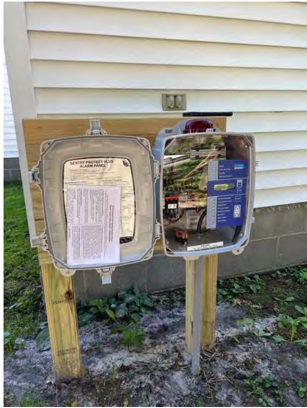
Town of Exmore (4400401): Control panel for grinder pump stations.
