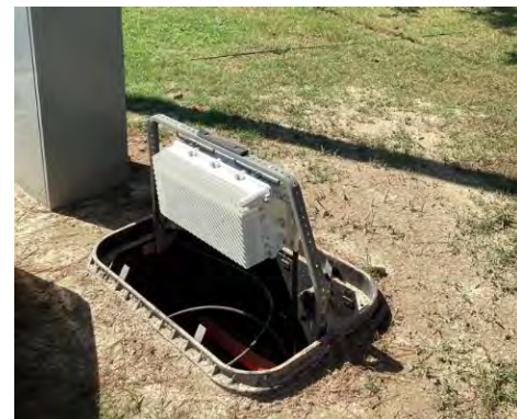
Cabinet Installation in Underground Fiber Construction in Hampton Roads Planning District Commission SLFRF Funded Project.
