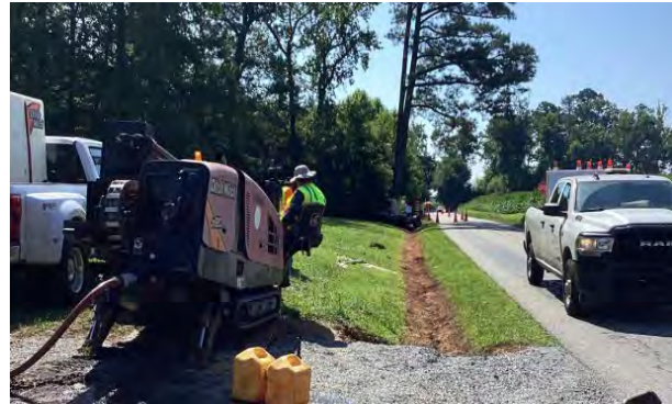
Mainline underground fiber optic construction in Hampton Roads Planning District Commission SLFRF Funded Project.
