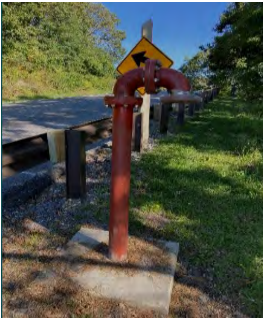
Nelson County (4400214): Last vent pipe that was installed as a part of ARPA project.
