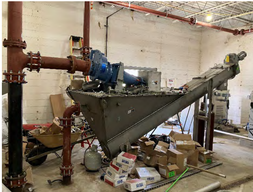
Wise County PSA (4400301): New preliminary treatment equipment for grit removal.
