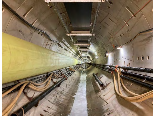
Alexandria Renew Enterprises (4400101): Portion of the Waterfront Tunnel constructed via the Tunnel Boring Machine.
